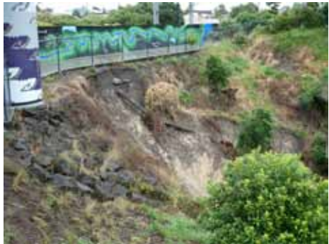
Photo (above): Railway Heritage Area slump
