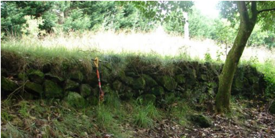
Plate 9. R11/2473 illustrating close proximity of a tree.
