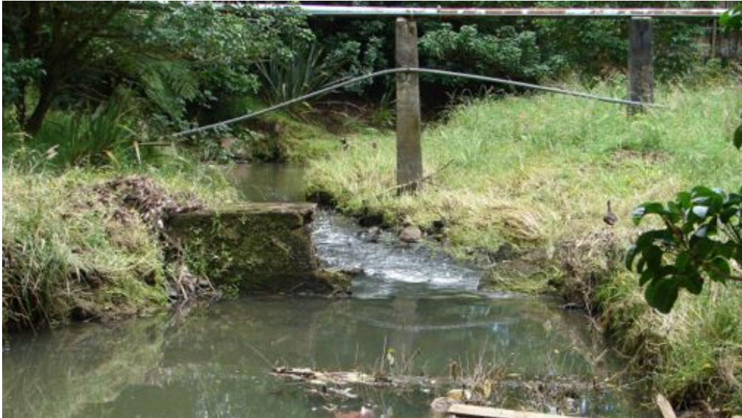
Plate 14. Remains of the crossing (dam?), showing relatively intact western side, the eastern side is discernibly collapsed on the right.
