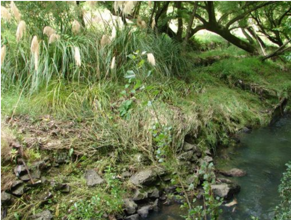
Plate 10. Toetoe above the stone bridge foundations, willows (background) over approach track to bridge, eastern side, these should be removed.
