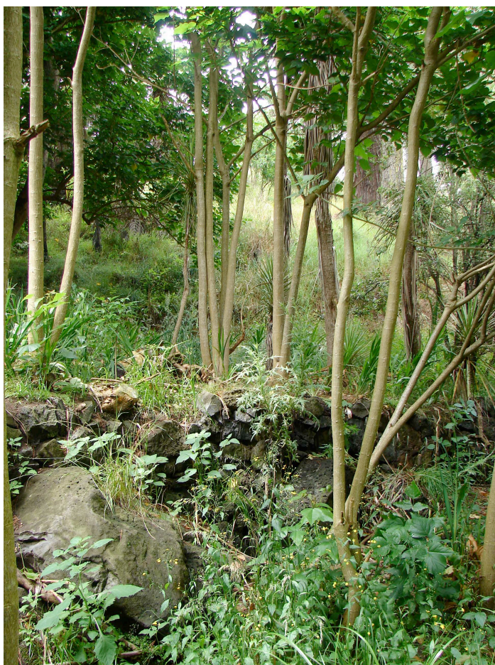
Plate 13. Young saplings growing in close proximity to the drystone retaining wall.
