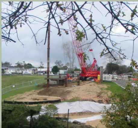
Left: Work has begun on the new Alford St Bridge, part of the Waterview Shared Path. Note that the Walkway in this area will be closed from July 2 nd for some months. Photo: W. John
