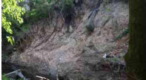
Photo (above): Slip around visible soakaway pipe
