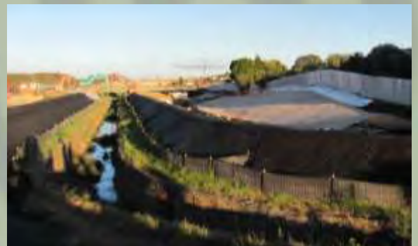
Above: The final portion of Oakley Creek to be realigned from a basalt channel (left) to a naturalised meander (right), with woolmat laid for erosion control in preparation for planting.
