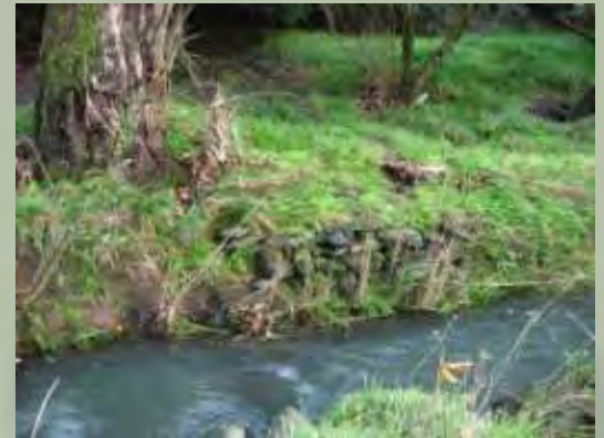
Above top: Remains of the old railway bridge; above: Remains of the old bridge below the BP petrol station. Photos: W. John
