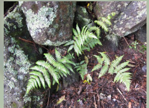
New growth on the gabion wall. Photos: W. John
