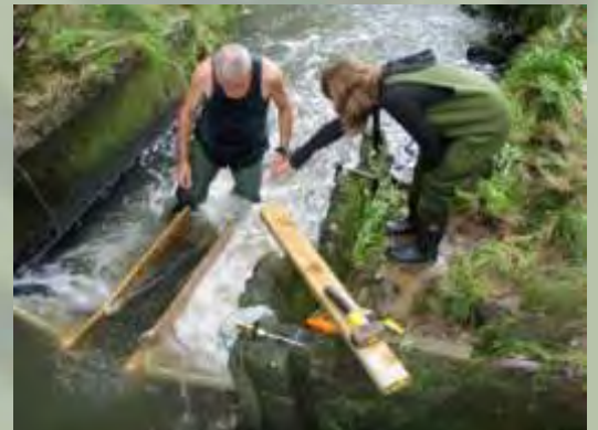
Pete Pattinson and Catriona Paterson installing the fish ladder at the Water Flow Monitoring Weir.
