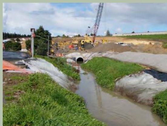
An Oakley Creek tributary is being put into a 372 m long culvert at the Maoro Rd Interchange on SH20 behind the Stoddard Rd shops - and there's much more of this type of work to come (see left). There were 145 short fin eels captured from here and released downstream into Oakley Creek at Alan Wood Reserve. Was there any research to determine the impact of this translocation? What other fauna and flora was left behind or destroyed? The high sediment load which can be seen in the photo was attributed by NZTA contractors to other housing developments upstream.
