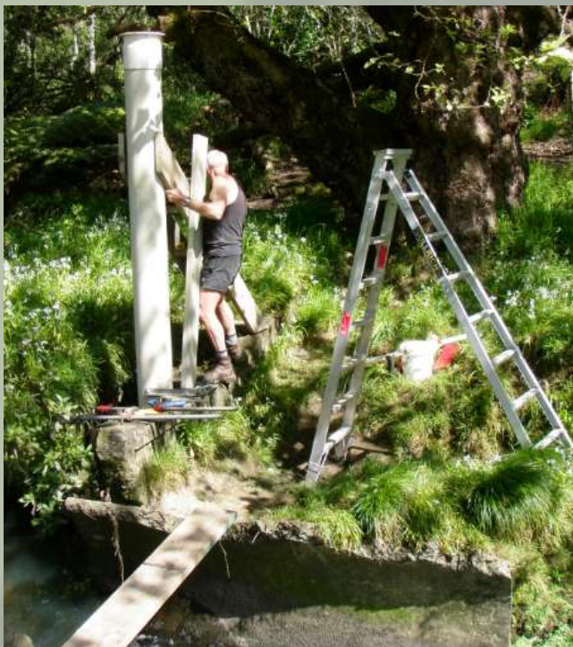
Pete Pattinson, NIWA , installed a replacement water flow monitor.
